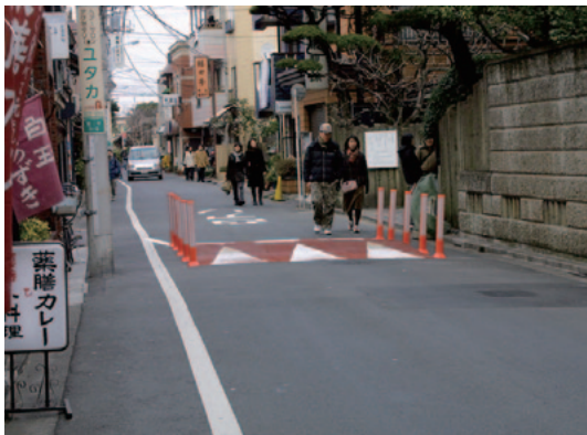
Figure 4. An experimentally installed rubber speed hump. Such experiments allow area residents to experience and evaluate impacts and effects. Noise and vibration is suppressed by the speed hump’s sinusoidal shape.
